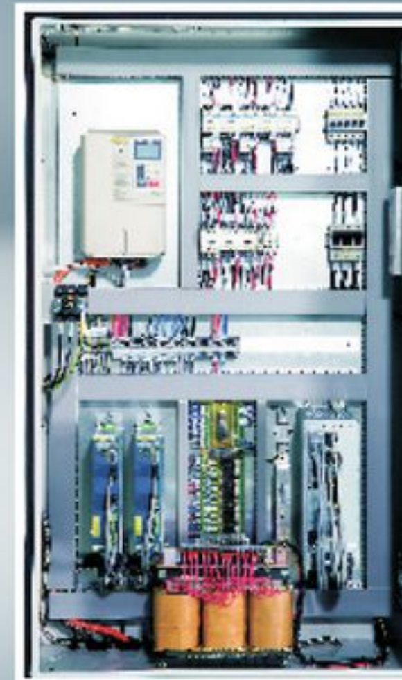
RIC-TC1800 ELECTRICAL CABINET FOR SPINDLE INVERTER MOTOR
