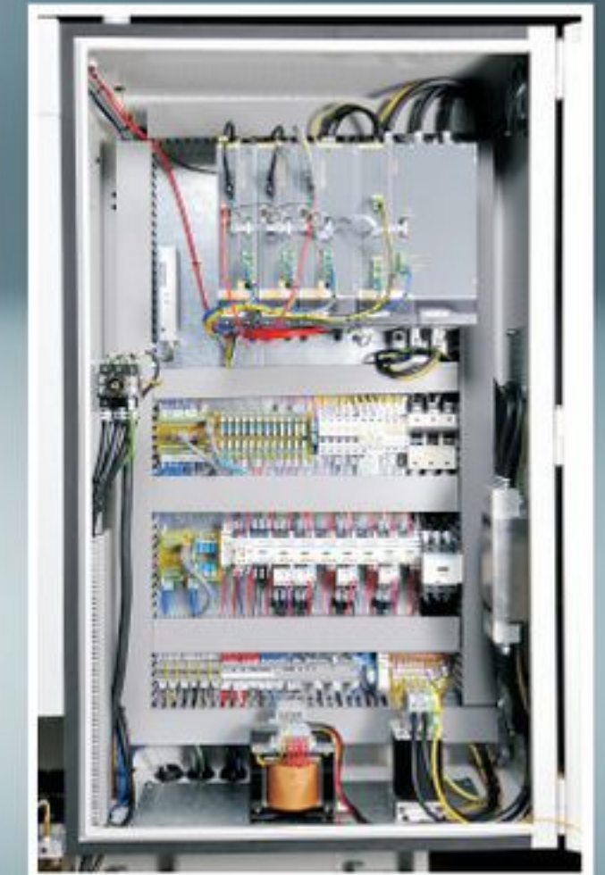
RIC-TC3300 ELECTRICAL CABINET FOR SPINDLE SERVO MOTOR
